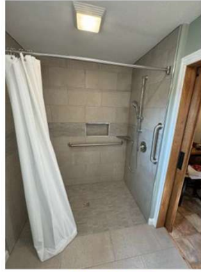
New Shower Grab Bars Handheld Shower
