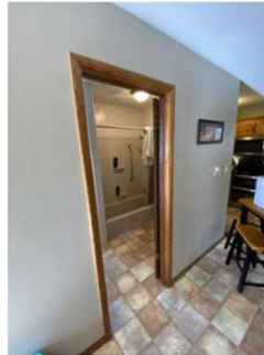
Doorway too narrow
